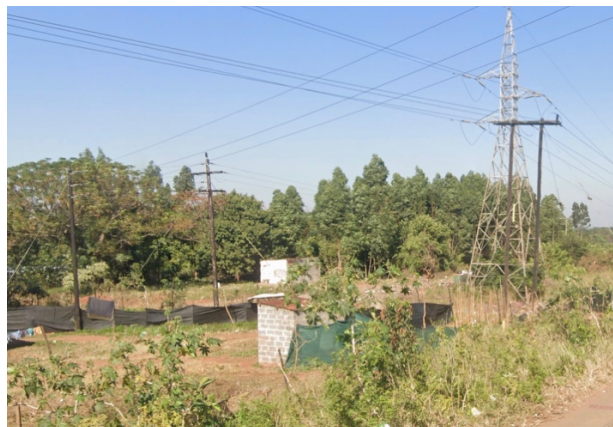
Existing Impala-Zircon 22kV powerline in Madlankala
